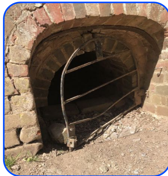
Damage to Grill and Brickwork
